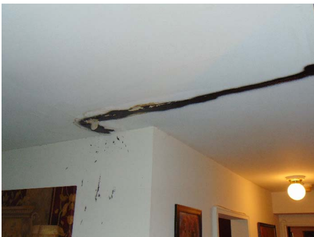
Water damaged ceiling materials
