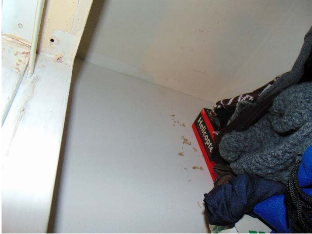
Impacted closet wall and ceiling
