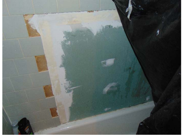
Incomplete shower wall (exposed drywall)
