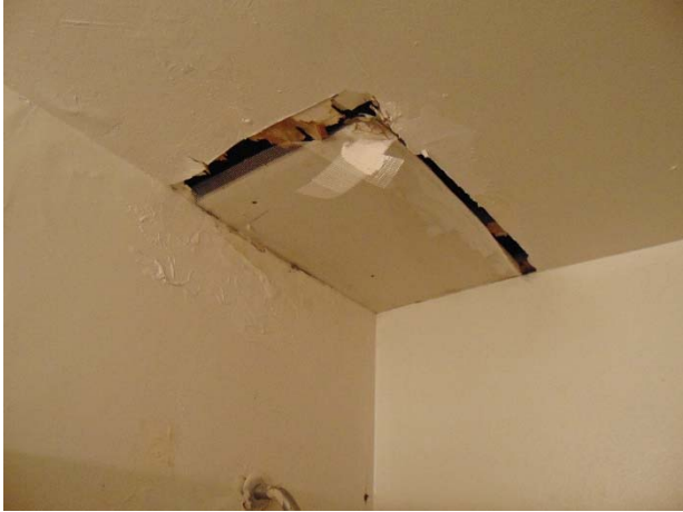
Impacted bathroom ceiling and wall
