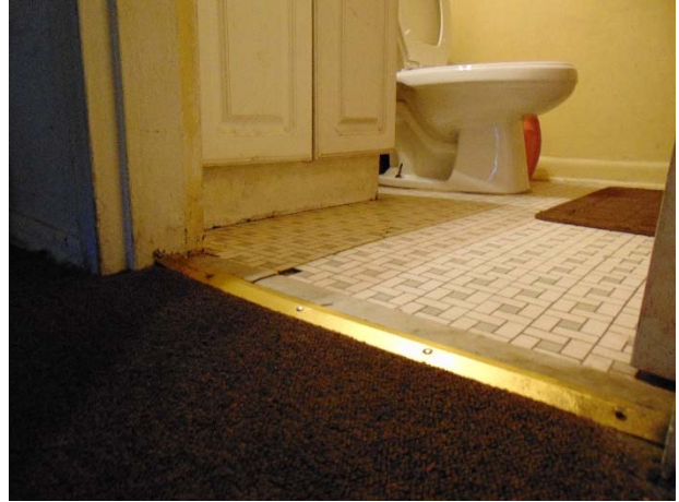
Visibly damaged bathroom flooring
