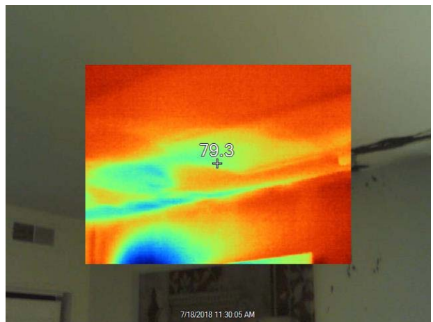
Active water intrusion into living room ceiling
