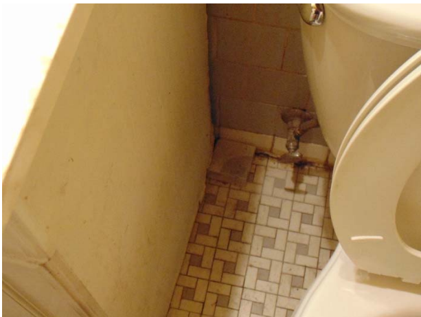
Visible mold growth and water damaged wall materials
