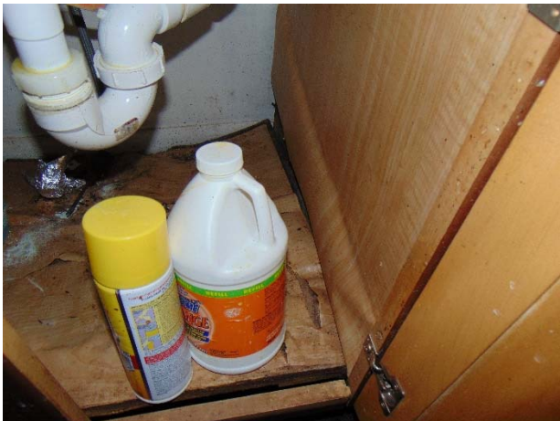
Visible mold growth on kitchen base cabinet
