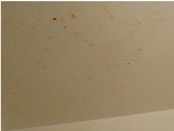
Wet bathroom ceiling and wall materials with visible mold growth
