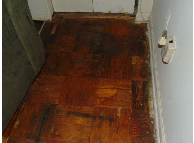
Visible mold growth and water damage hallway flooring
