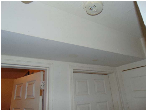
Impacted area in hallway
