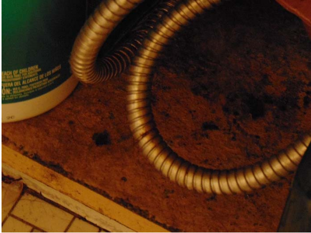
Visible mold growth inside bathroom vanity
