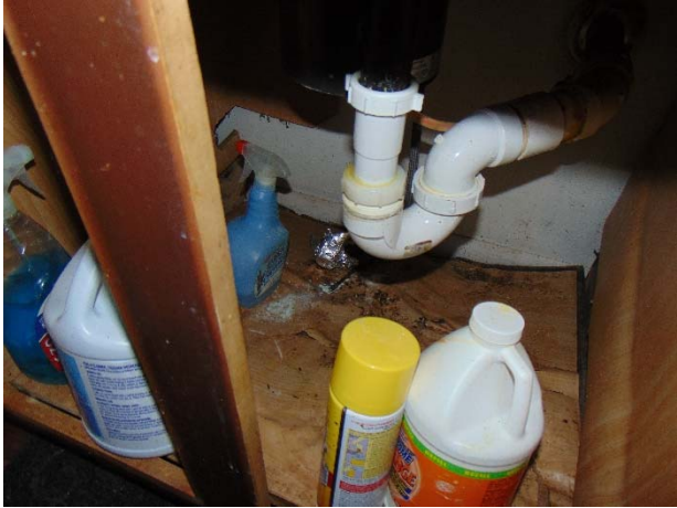
Kitchen base cabinet water damage and visible mold growth on wall materials behind
