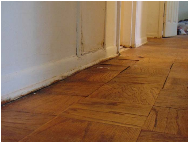
Impacted hallway flooring
