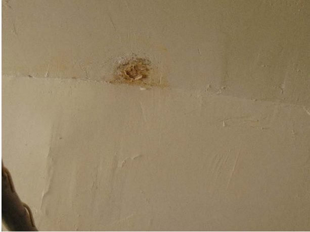
Wet bathroom ceiling and mold growth
